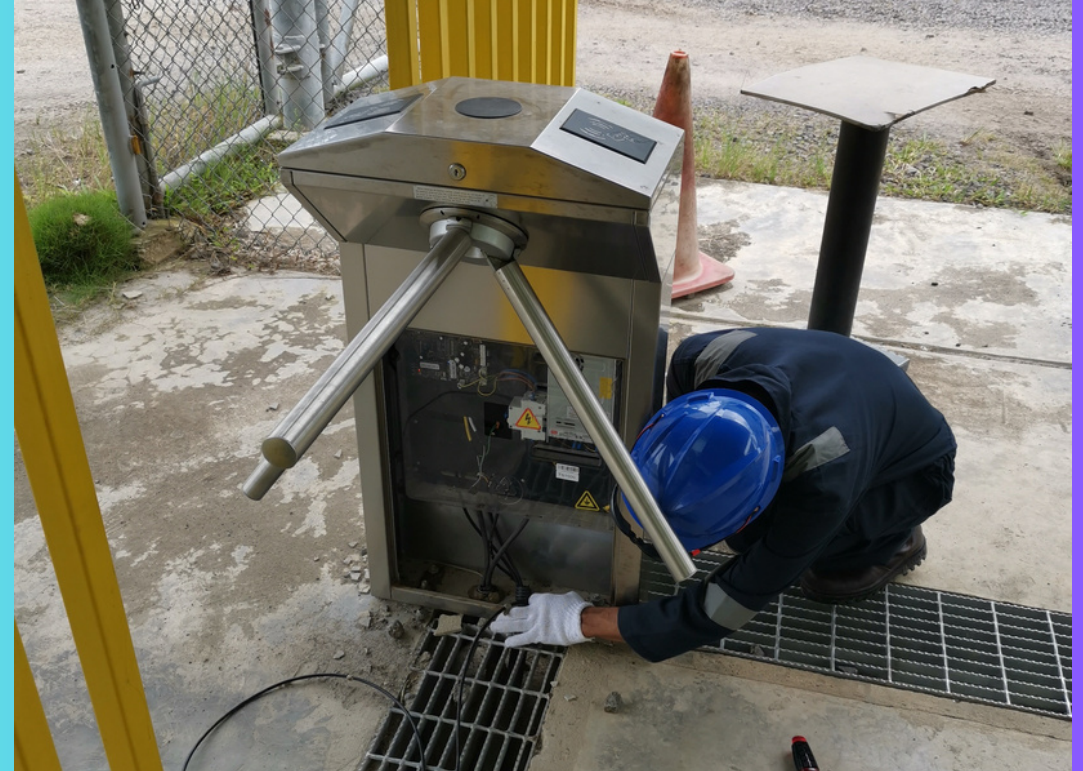
Access Control Pertamina Jambi Merang
