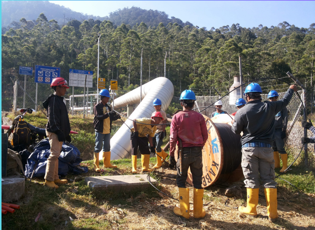
Fiber Optic Instalation StarEnergy Geothermal
